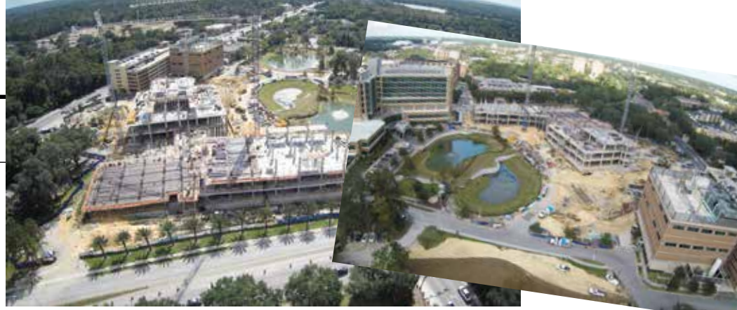
These stills, taken from drone footage, show the construction progress on the new UF Health Heart & Vascular Hospital and the UF Health Neuromedicine Hospital.
